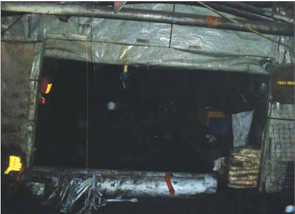
Figure 16.3: View of the upper FAB looking inside 79
