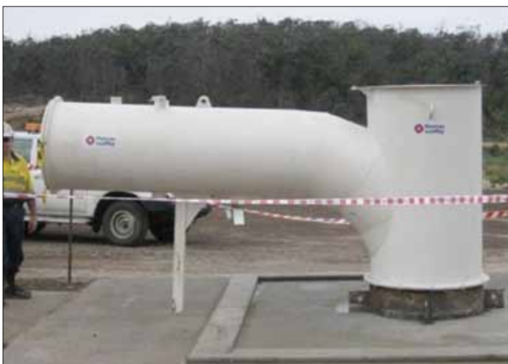
Figure 33.6: Inertisation connection facilities
