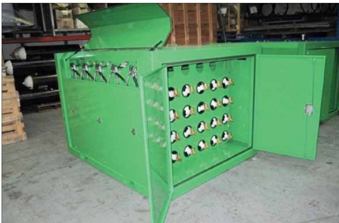
Figure 33.3: Recharge station for compressed air breathing apparatus
